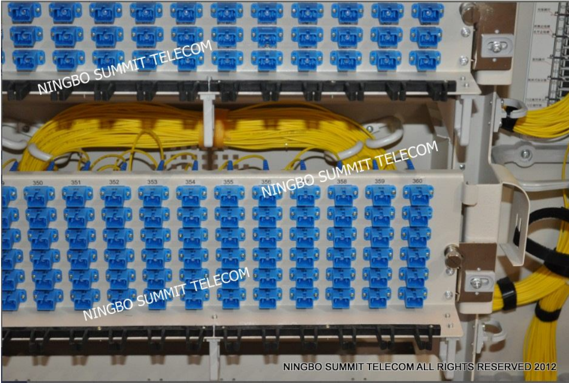
Pacth Tray on right side for fiber patching and termination.
