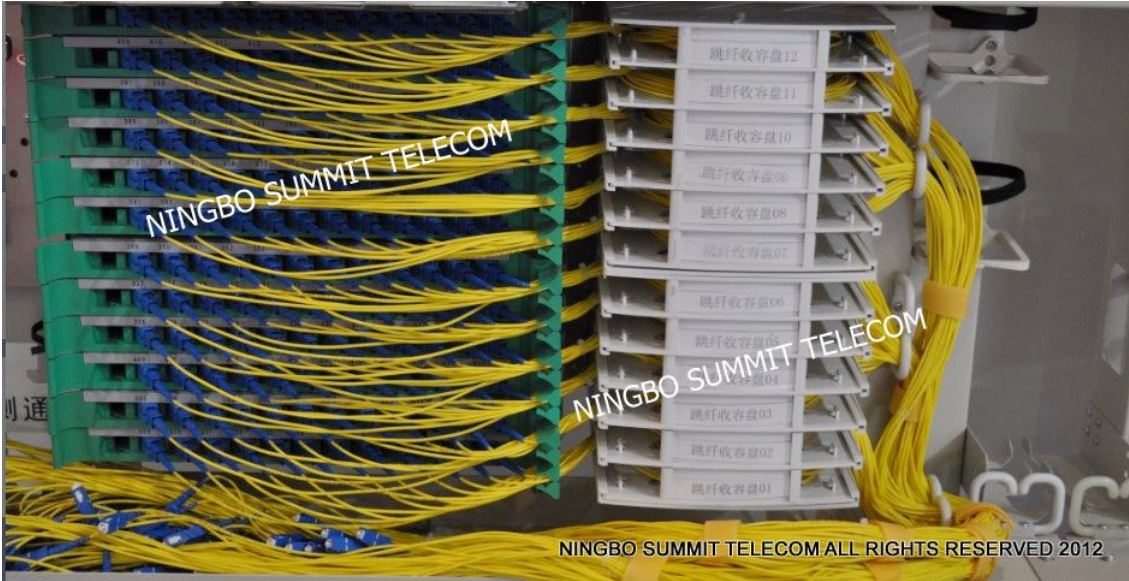
Splice Patch Tray on left side for fiber splicing patching.
