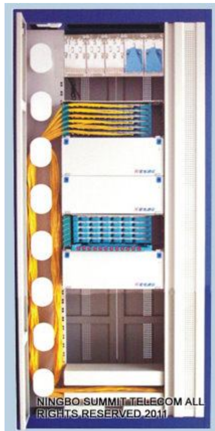
Picture1 Fiber Optic Distribution Frame STODF01
