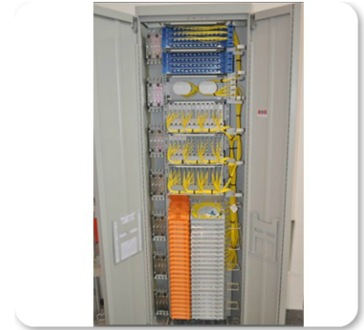
19" Fiber Optic Distribution Frame With PLC
